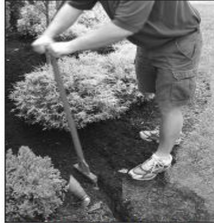
Pushing the tool back and forth widens the trench and creates a channel for the wire.
