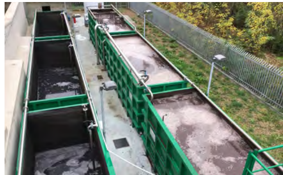
New wastewater treatment at Pontassieve
