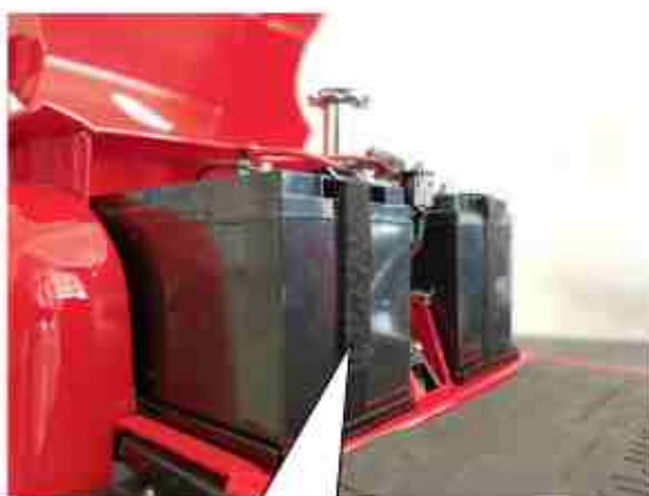
Battery tie down straps
