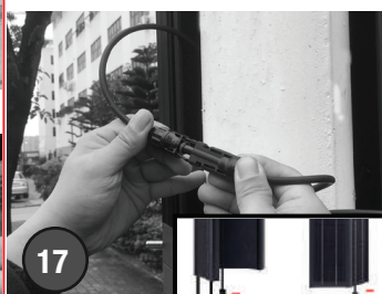
17 Connect the first module to the second module by MC4 plugs directly. Plug in, easy operation.
