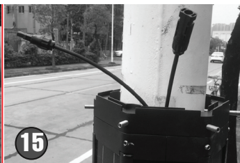
15 Make sure the two MC4 cables are outside through the third brackets. (Ready to install the next modules.)
