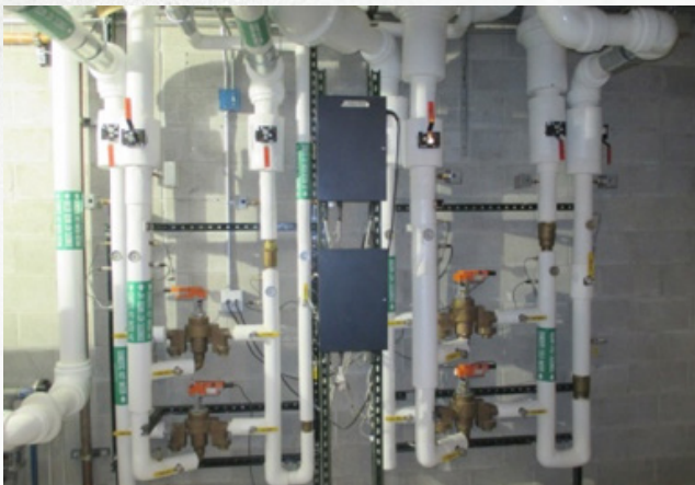
Acorn BASyC system that features two SFMMV supply fixtures, installed at Northwestern Medicines - Lake Forest Hospital
