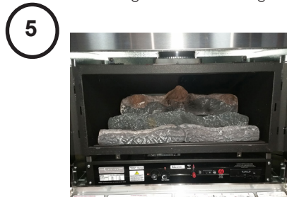
Fit the remaining log over the pins and the logset is complete!
