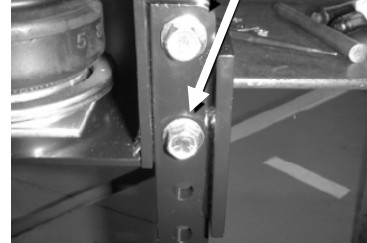
Figure 4.28 Bolt head on the riser leg
