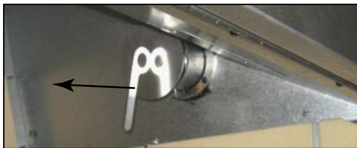
Figure 4 Outside Air Tube Opened
