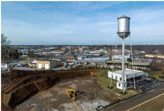
Developers say an existing water tower above the distillery will be wrapped to look like a bourbon barrel with the Turner Commons and RD1 Spirits logos and will light up at night. Ryan C. Hermens rhermens@herald-leader.com
