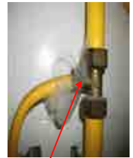
Bubbles indicate gas leak
