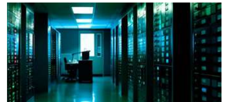
IN SERVER CENTERS
