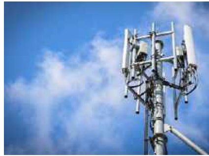
MOBILE BASE STATION
