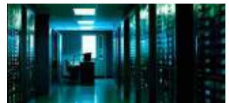
IN SERVER CENTERS
