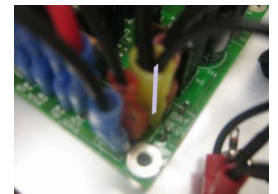
e. Battery Negative Wire (shown in light purple).
