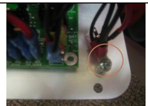
g. Ground wires from feed and battery negative black wire (shown in light brown )
