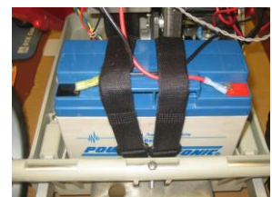
Battery Terminal Wires
