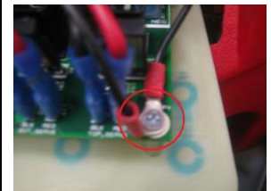
Ground Wire Connection Screw (marked in red).
