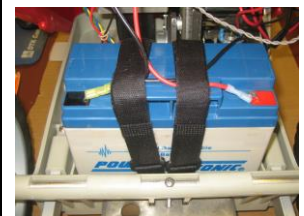
Battery Terminal Wires
