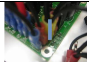
f. Battery Negative wire from battery
