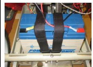
Battery Terminal Wires
