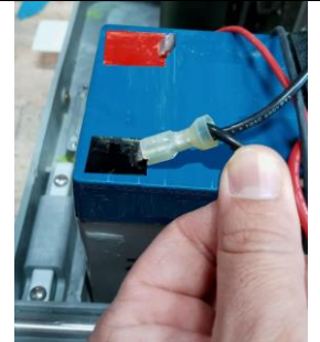
Negative wire being connected to Battery.
