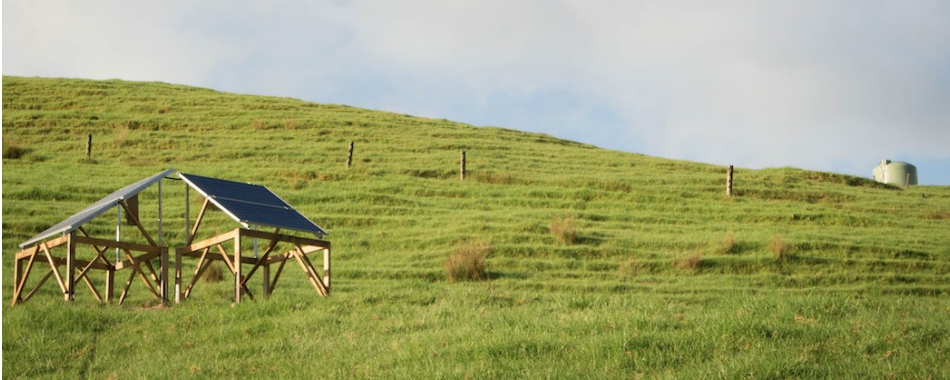
1080W of PV on movable frames (540W per frame)
