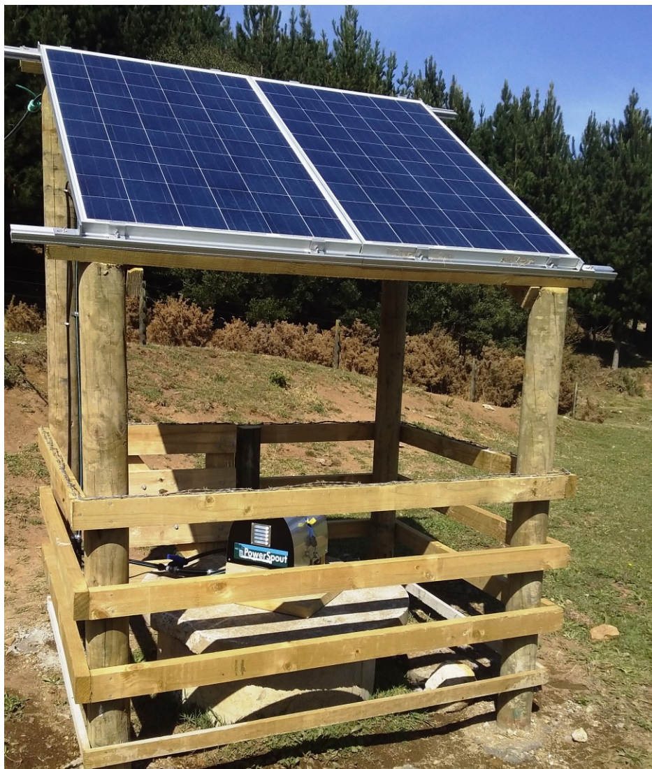
2 panel React pump ground mounted above a shallow farm well
