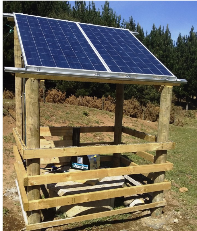
Typical installed PV array (there are many ways to install solar PV)
