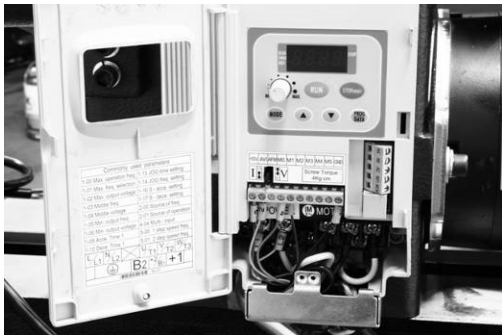
VFD with cover open
