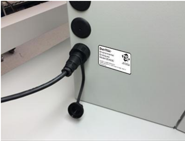
Figure 21: DC Cable from Solar Battery to Environmental Enclosure
