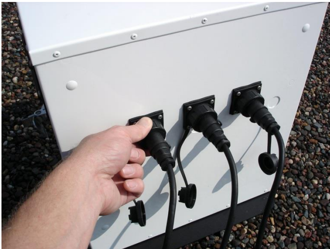
Figure 12: Connect Power from the Solar Cell Power System to the Environmental Enclosure
