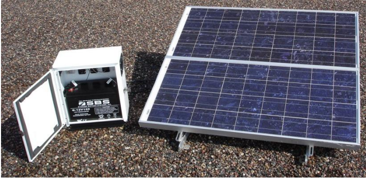
Figure 1: Solar Cell Power System
