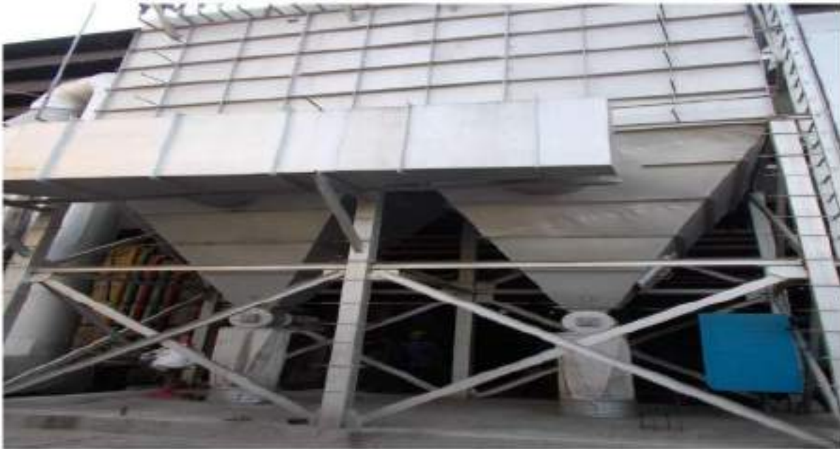
Figure - Baghouse Filter
