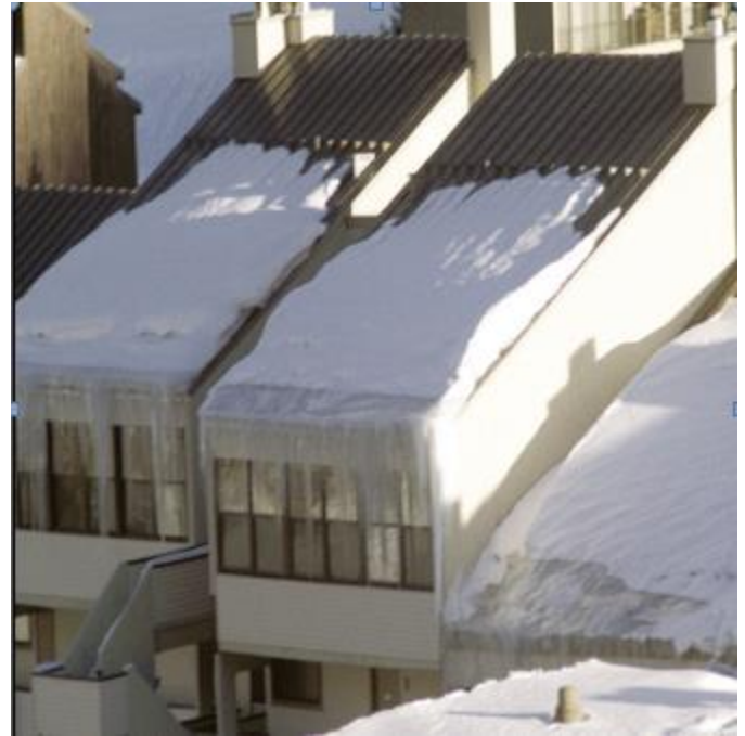
Figure 6B: Ice dams create unintentional snow retention
