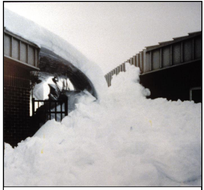
Figure 5: Sudden release of roof snow
