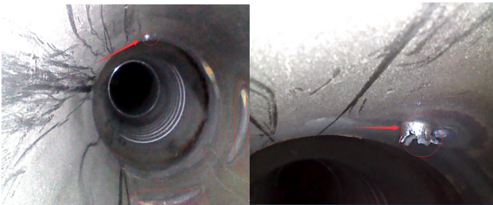
The inside flaw of the exhaust pipe
