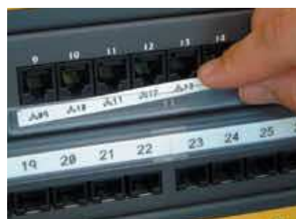
Punch block & patch panel labels
