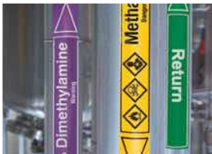
Pipe & valve marking
