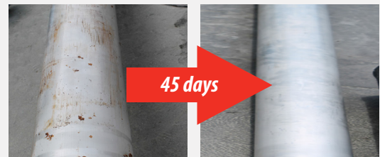
Overfill preventer in service 1 year Granite Rock, Santa Cruz, CA
