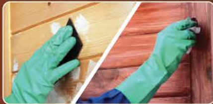
SCUFF WITH SAND PAPER dust it off, Apply 1 st coat of AWC
