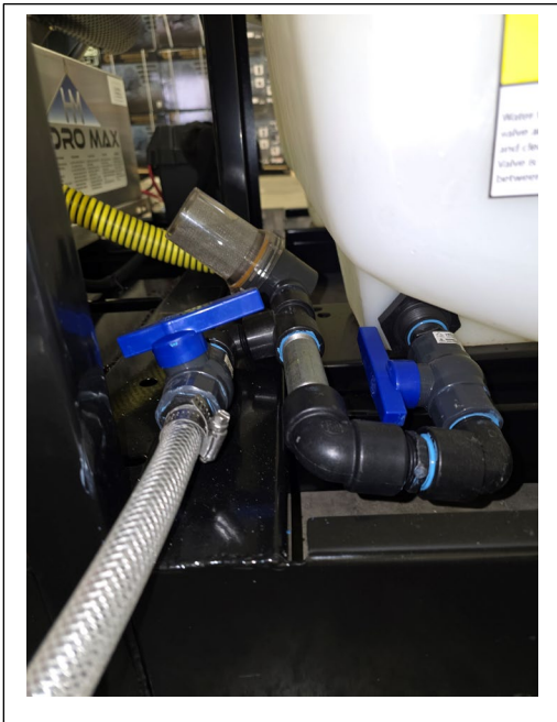
Tank valve plumbing w/ secondary feed line installed. Tank valve shown in the open position. Secondary line should be closed for normal operation.
