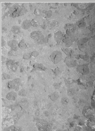
Localised corrosion for high levels of salt
