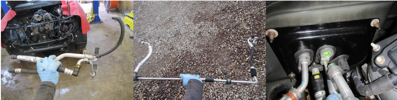
Step 8: Remove water lines, ensure cooling system is empty and evap system as well
