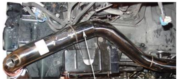
LHS Discharge Duct
