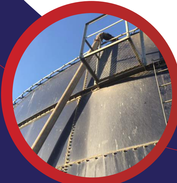
Slurry Tank at Winnifred Colony Dairy Medicine Hat, AB CA. Continuously applied, no sludge build up problems over yrs.
