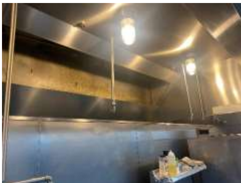
Kitchen hood, behind the filters prior to cleaning
