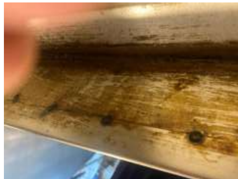
Close up of area behind hood filters
