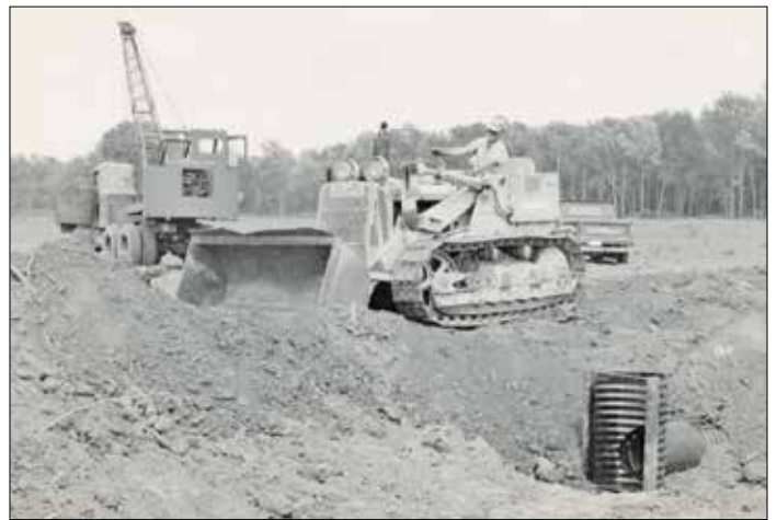
Maintenance employee Franklin Robinson building a field impoundment dike with our crawler-mounted front end loader. Flashboard riser in lower right of photo.
