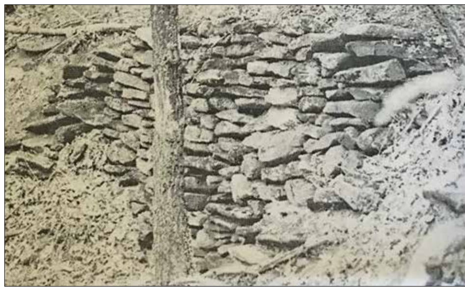
A photo of old stacked stone walls that ran along parts of the old CCC road. SMOKE SIGNALS SEPTEMBER 1997
