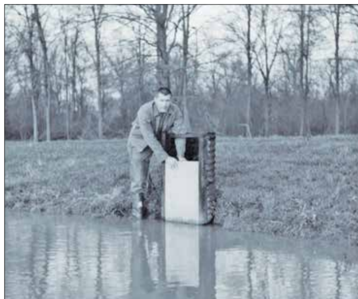
McDaniel slipping flashboards into the riser portion of a completed field impoundment. Impoundment will hold water up to the top board before the overflow exits out the horizontal portion of the structure.
