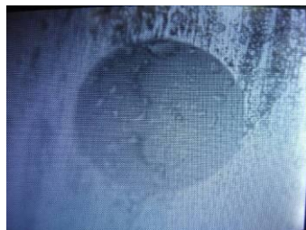
Dirty: Cleaning required
