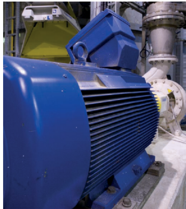
Pump drives in a paper machine
