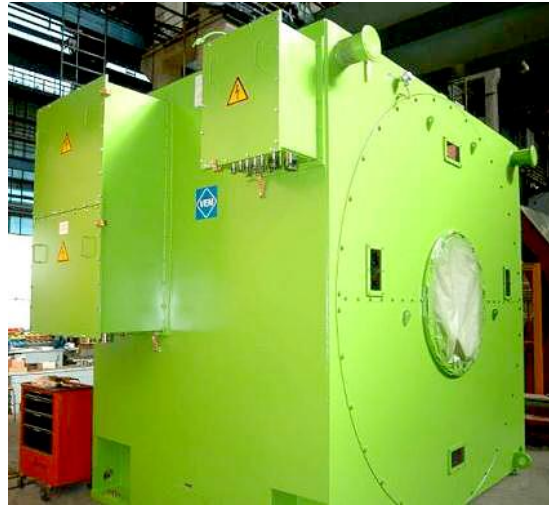
Wärtsilä SAM Electronics GmbH, container ship for Hapag Lloyd HHI shipyard, Korea
