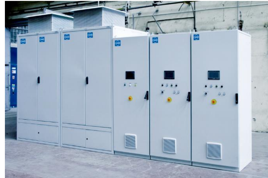
Type: LCI (Load Commutated Inverter) For polyethylene (LDPE) plant/high-pressure process For synchronous motor 23,000 kW, 11,000 V, 200 r.p.m.
