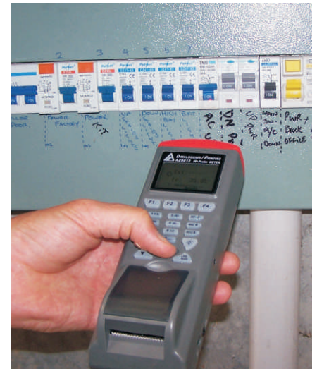
Typical use on switchboard
