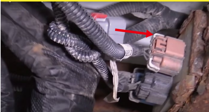
13. Plug into the junction box.
