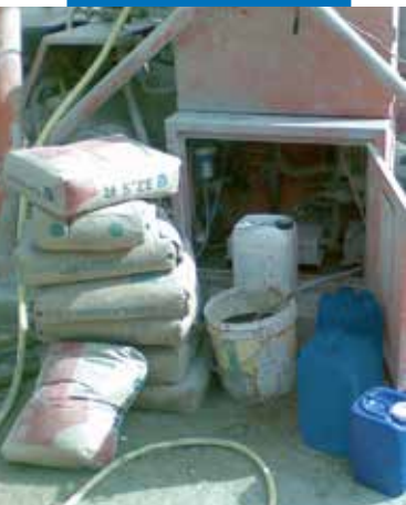
Mechanical system for metering Mapescreed 704
