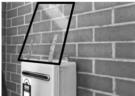
A rigid sheet of clear polycarbonate installed on an angle up to the wall preventing the cat from using the gas unit as a platform.
