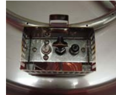
Top View- note next to burner
