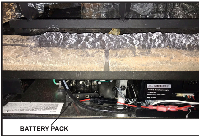
Figure 6.3 Battery Pack Installed
