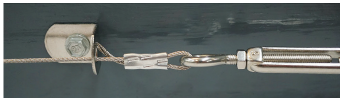
Guide wire fed through eyelets to create a wire framework for attachment to netting.
