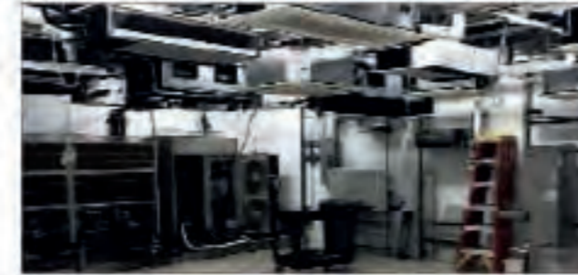
LG Air Conditioning Academy
