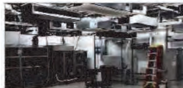
LG Air Conditioning Academy
