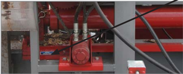
Shown Here: Splitter Cylinder Base
