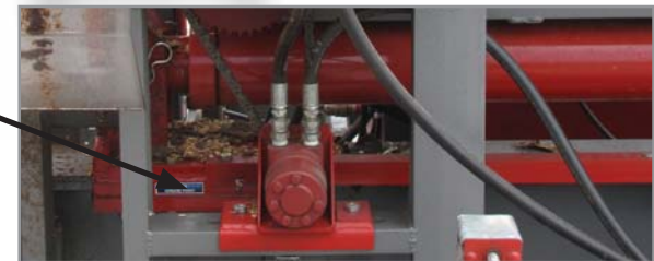
Shown Here: Splitter Cylinder Base
